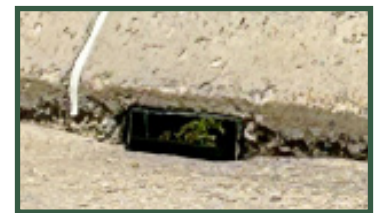
A simple drop through scupper at the base of a concrete barrier that has been cleaned and maintained. Photo: ISMF LLC
