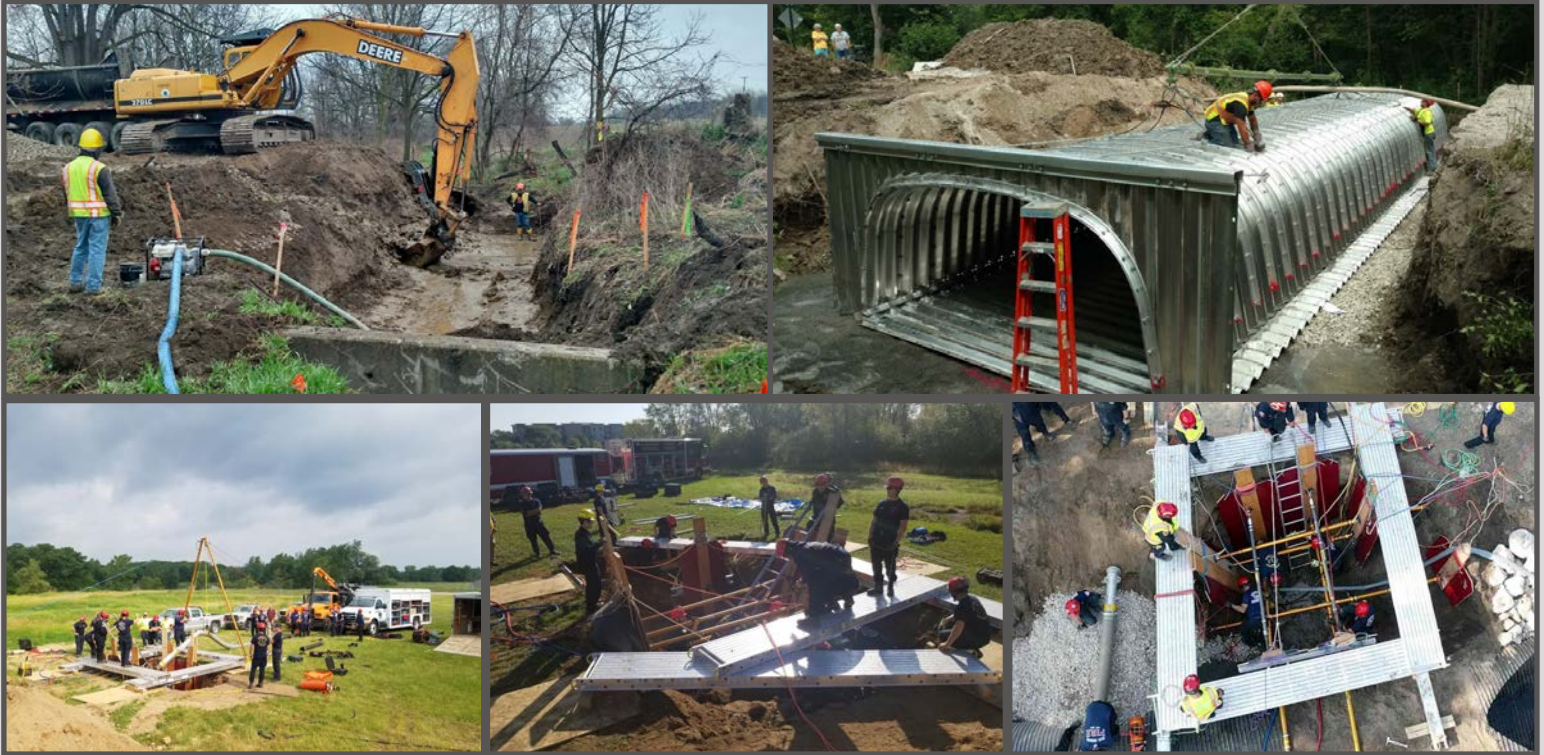
Top row: Washtenaw CRC's trenching and excavation for culvert installations. Bottom row: Washtenaw County tech rescue team practicing a trench rescue at Washtenaw CRC. (Photos: Courtesy of Washtenaw CRC)
