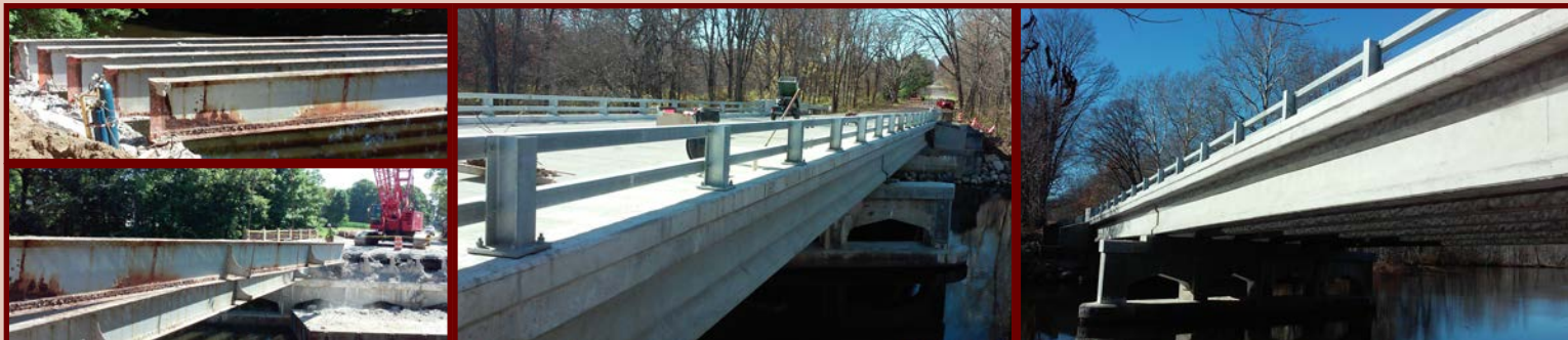
108th Street bridge project over Thornapple River: left top – beam ends in the worst condition before project; left bottom – removing beams with crane during project; center – near-finished condition; right – finished condition (photos courtesy of Kent CRC)
