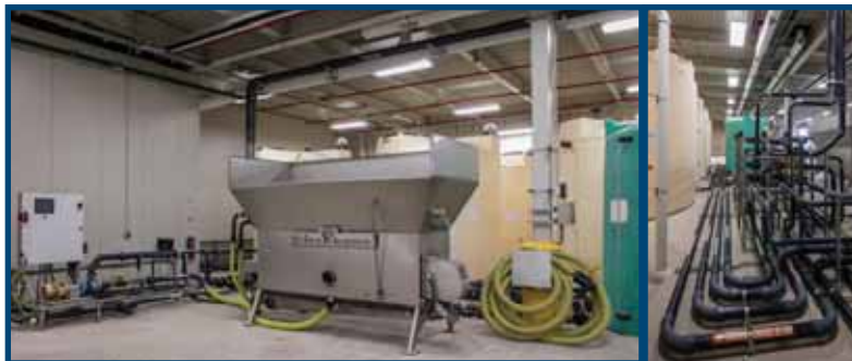
Brine-making facility at City of Farmington Hills (Photos courtesy of City of Farmington Hills DPW)
