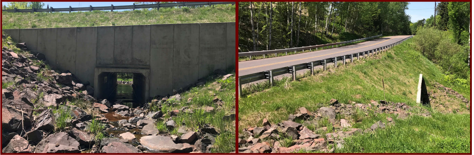
Restored culvert crossing, one of Phil Strong's projects following Gogebic County's 2016 storm event. The new culvert is an 8-by-6-foot, 20-foot-deep precast concrete box culvert. (Photos: Courtesy of Gogebic CRC)
