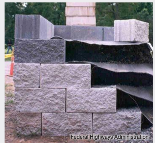
A cross section of a GRS-IBS abutment. The outward-facing brick is a non-structural veneer that protects the inner material.
